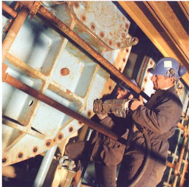
A Removal of end plate on sea water condensers at Hunterston A.
